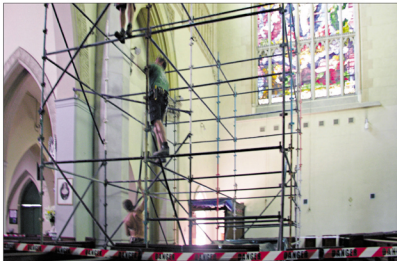
Up she goes: Workers erect scaffolding inside St Mary's Cathedral in Perth so that architectural study of its internal construction can be conducted.
