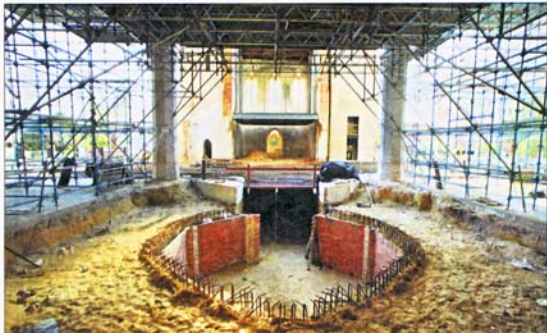
New beginning: An underground crypt is being built during renovation work on St Mary's Cathedral. Pictures Steve Ferrer
